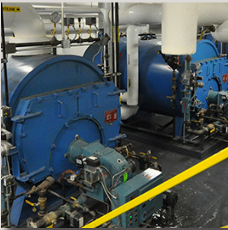
Maria Regina High School - new boilers infrastructure project.
